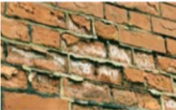
Photo illustrating an area of brickwork NOT treated with Waterstop
