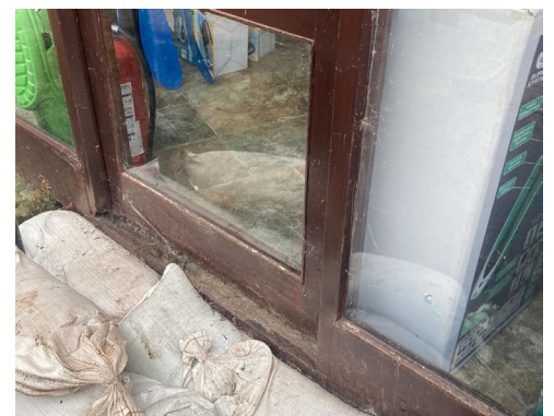
Photo showing previous timber doors with sandbags post flood event
